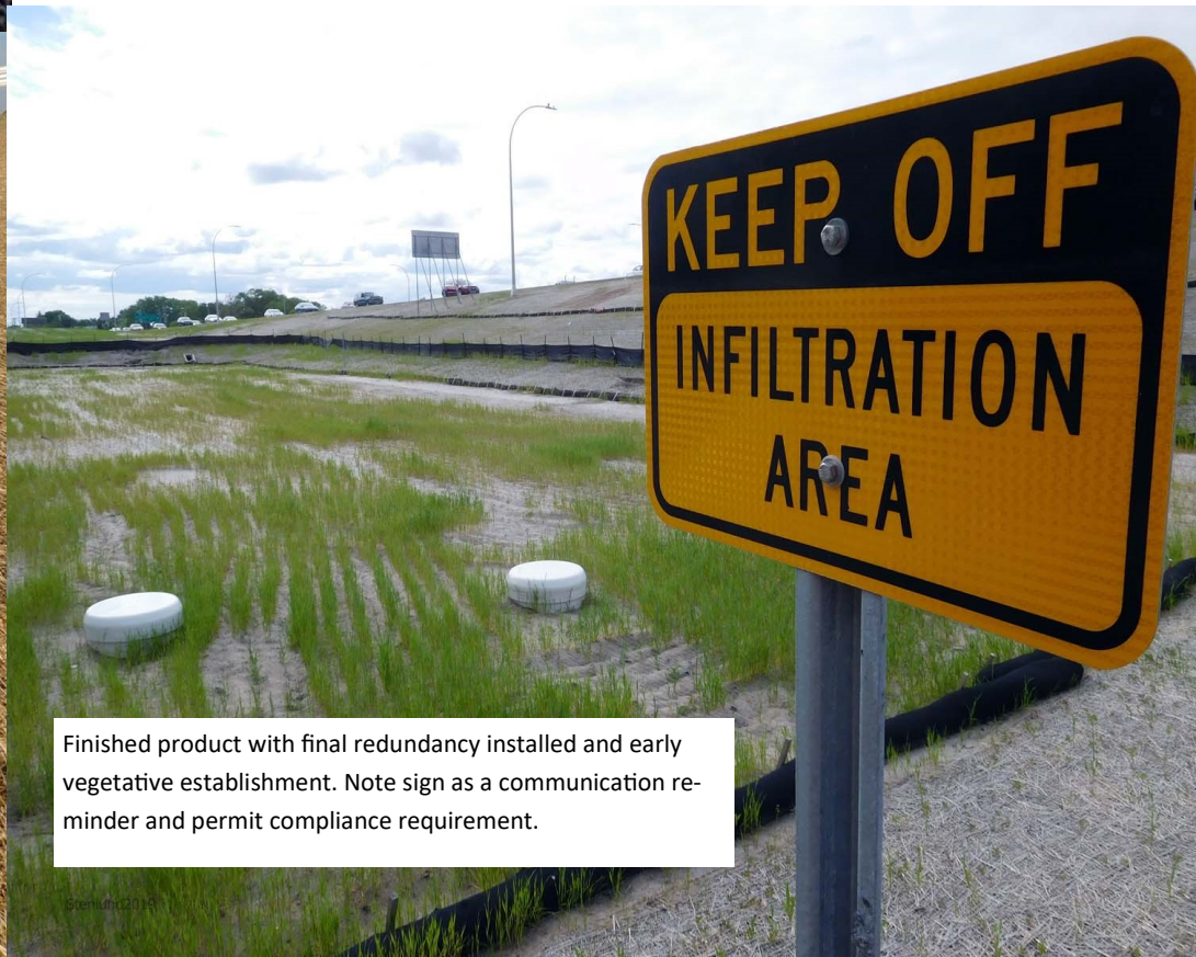
All sediment control BMPs require maintenance. Redundant perimeter control is no exception. Continue monitoring and documenting visual inspections (1) 48 hour draw-down, (2) sediment loading, (3) erosion, and (4) vegetation establishment for diversity and density. Perform corrective actions immediately to preserve function and integrity.
