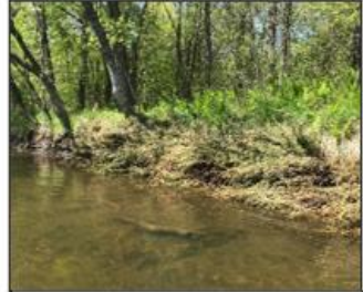
The cedar trees were anchored parallel to the shoreline and willow stakes were added between the trees. Willow stakes will grow and spread into a shrub grove to provide long lasting bank protection and habitat.
