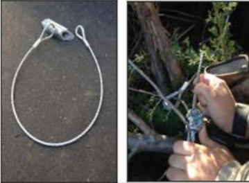
Cedar trees were tied together using cable and cable clips. The trees were then secured to the riverbank using a duckbill anchor with the trunks facing upstream to divert the flow of water away from the bank.
