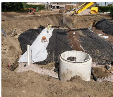
The stormwater treatment practices will include the installation of a StormTech underground stormwater filtration system along with a dozen sump manholes with baffles.
