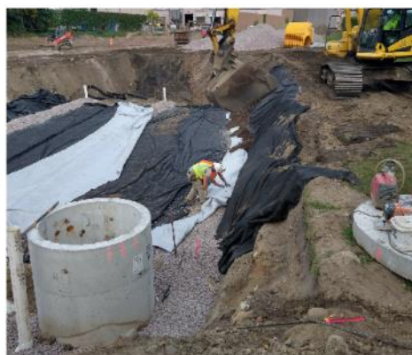
The project goal was to direct dirty stormwater that runs off from yards and city streets into this underground stormwater filtration system instead of letting it continue to go untreated into the Mississippi River as it has in the past.
